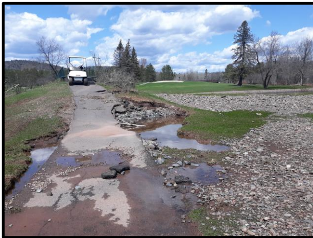
Photo 3: Damage to Cart Paths
